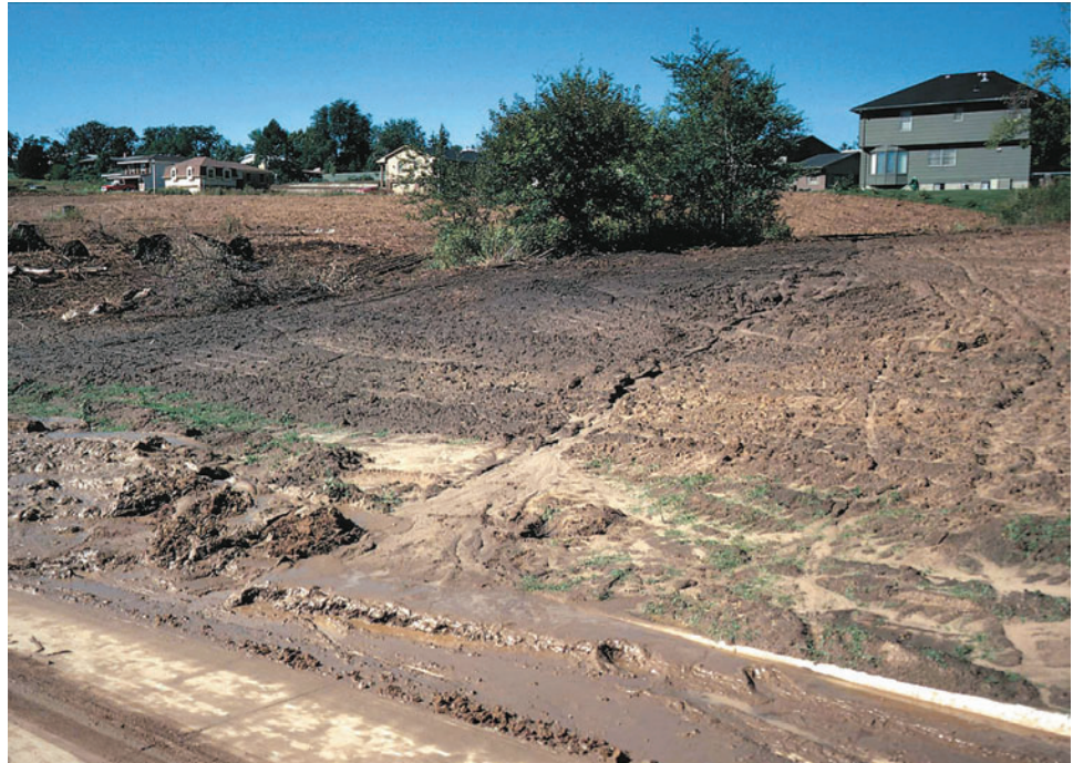
Figure 20. Sediment Runoff During Construction: What Should Be Prevented
