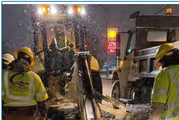
CAW crews working through the night to repair main leaks resulting from the extreme weather event in February 2021.
