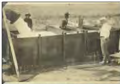
Treatment Water Well E – April 1925 – Arkansas Water Company employees try to figure out how to stop the leak.
